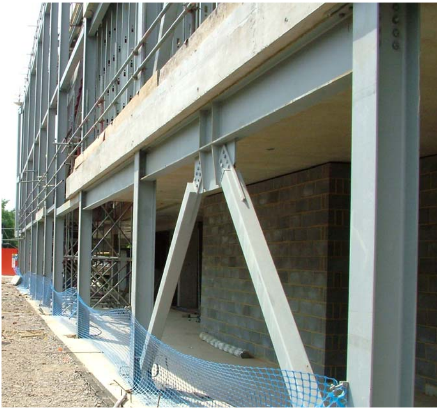
Structural steelwork ready for a glass façade on the new Woking Galleries, Woking Museum and Arts & Crafts building.
